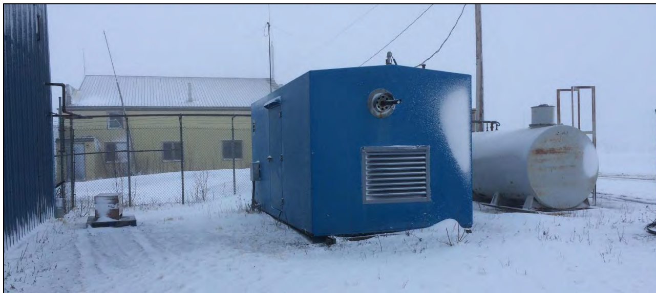
Figure 5-1 Fuel tank for the emergency generator, equipment enclosure with the electric enclosure and emergency generator.
