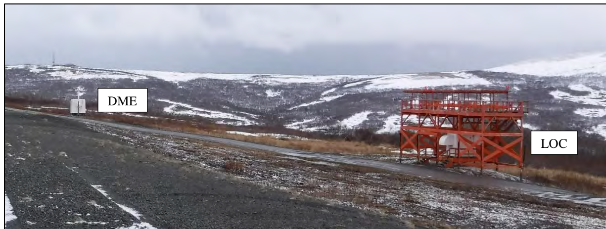
Figure 1-11 Runway 17 Localizer and DME, looking east
